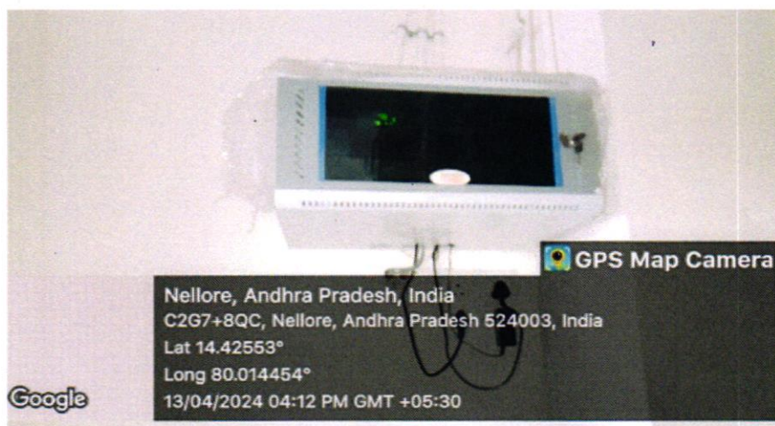
LAN at 2 nd Floor
